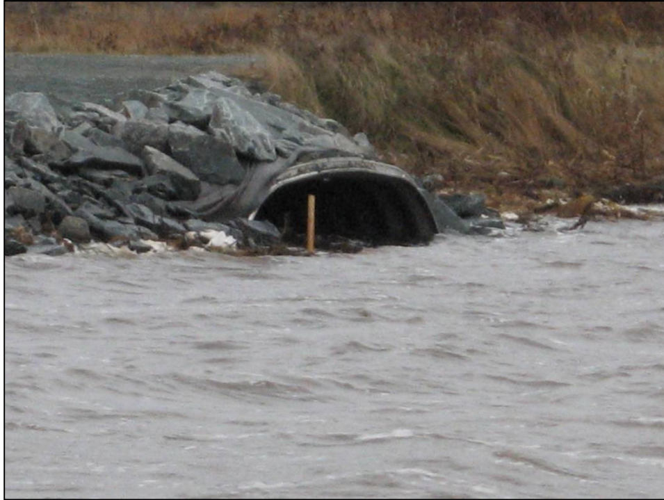
Figure 6 Downstream (lake side) end of the new culvert installed in the Trans Canada Trail to reconnect LT to the greater Lawrencetown Lake tidal system. Photograph by T. Bowron 2007.
