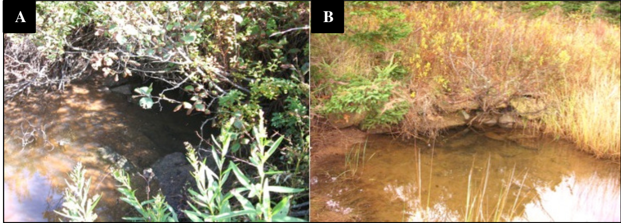
Figure 9 Upstream (A) and downstream (B) ends of the original concrete culvert at LT. Photograph by CBWES Inc. 2006.
